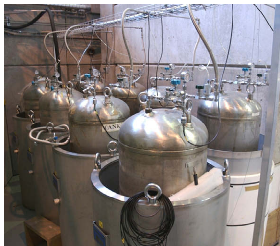
Fig. 2. GXe storage tank.
